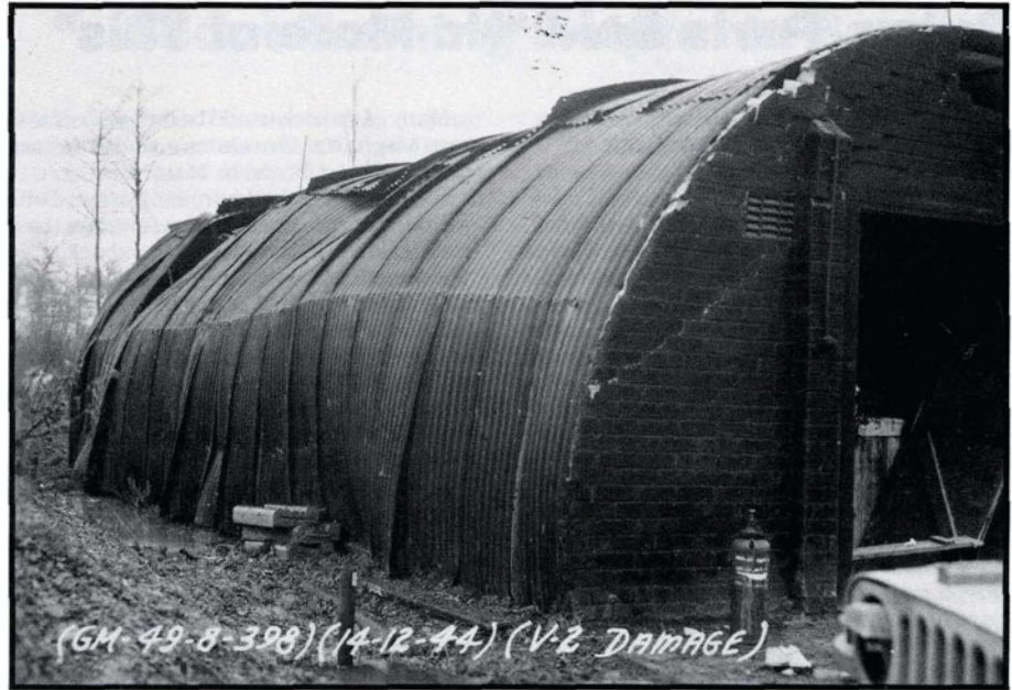
ONE OF 13 DAMAGED ORDNANCE HUTS
